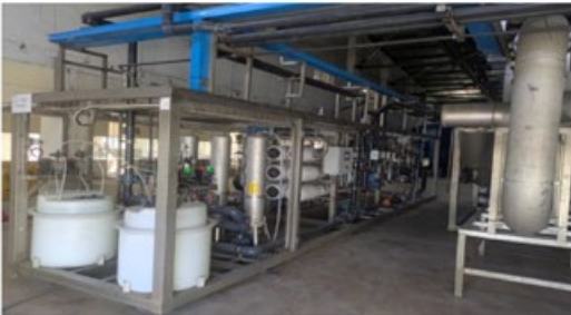
4th-Stage RO Installation – VFB
